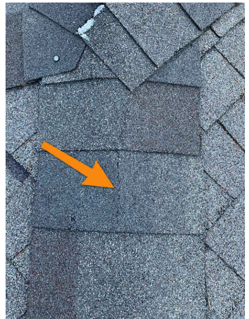
Cracked ridge shingles - multiple places
